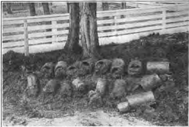
Fig. 65. A tile drain which became completely obstructed by roots from a willow tree.
