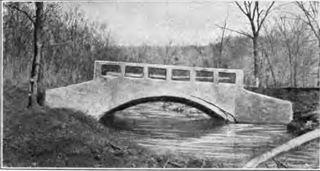
Fig. 98. A concrete bridge which failed on account of the foundation.
