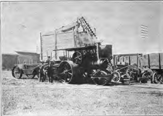
Fig. 93. Stone crushing plant. A three-wheeled steam roller and a dump wagon are shown in the foreground.
